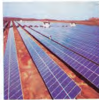
2.5 MW Solar PV, in Sal, Cape Verde Commissioned October 1, 2010
