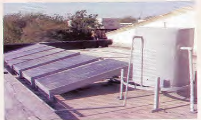
Pilot Water Heater at UDUTH by SERC, Sokoto
