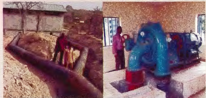
Penstock bifurcation into the 150 kW power house at Waya Dam, Bauchi State
