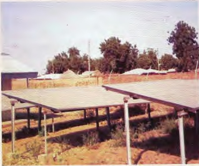
Solar PV mini-grid in a village in Sokoto, Sokoto State
