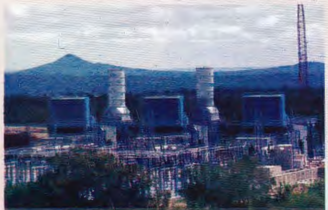
414 MW Natural Gas Fired Power Plant, Geregu, Kogi State - NIPP
